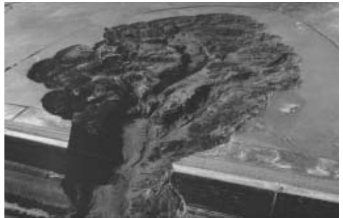
Figure 1 Hourglass shape of Merriespruit tailings dam breach, South Africa (Courtesy of Professor Andre Fourie). The 31-m high tailings dam was overtopped by rainfall–runoff and failed in the night of 22 February 1994.
