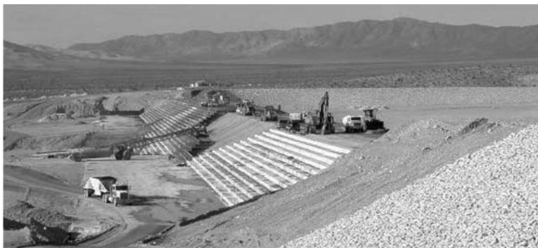
Figure 1. Stepped overflow protection system for a detention basin in west Las Vegas under construction (Courtesy of M.R. DELCAU and USACE-LA District).
