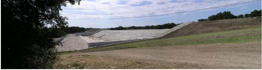
Fig. 1 Stepped spillway of Salado Creek Dam Site 15R (Courtesy of Craig SAVELA, USDA-NRCS-NDCSMC)—Roller compacted concrete construction, \theta = 21.8^\circ , h = 0.61 m
