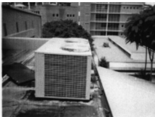
Air Conditioner on Roof Top
