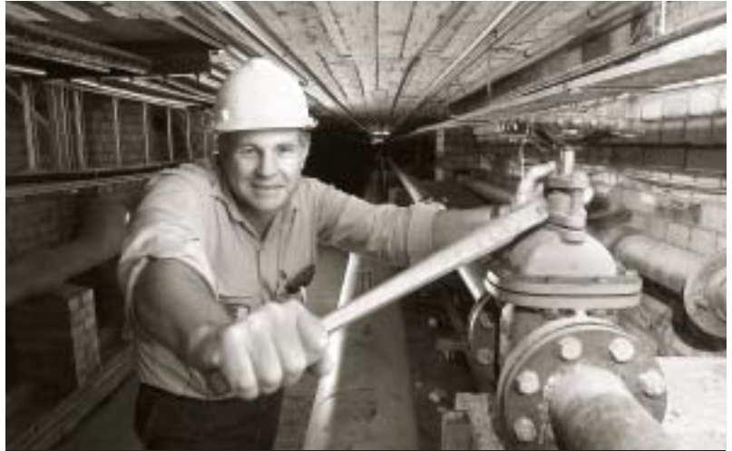
Alan Abbot (Property and Facilities) helps install specialised ventilation systems in the tunnels below the Great Court. The tunnels house cables and pipes servicing facilities ranging from IT to air conditioning.
