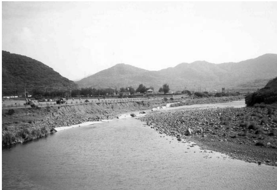
River bank erosion at Chenchung, PingTung county, Taiwan about 5 km upstream of the river mouth in December 1999. View from the right bank looking upstream.
